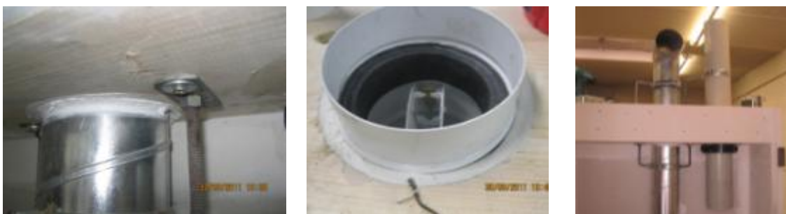
Figure 91: Rigid fastening of the ventilation pipe in the wood floor (left), fire protection closure based on intumescent materials with closing element FLI-VE (center), installation in sample body (right)
