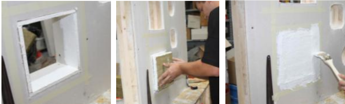
Figure 83: Installation of the soft partition in a sample body (left: reveal covering center: Installation of the mineral fiberboards that is coated on its edges, right: Overcoating of surface beyond the edge of 20mm)
