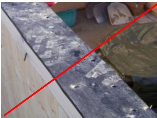
Figure 65: Inadmissible fastening of the elastic padding support using nails
