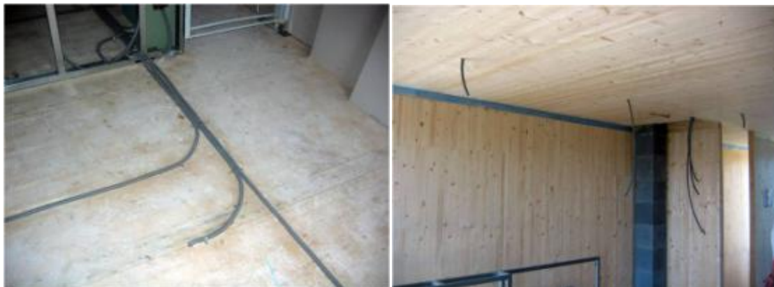
Figure 37: Laying of electric cables is to be executed in an airtight way for visible cross-laminated timber floors
