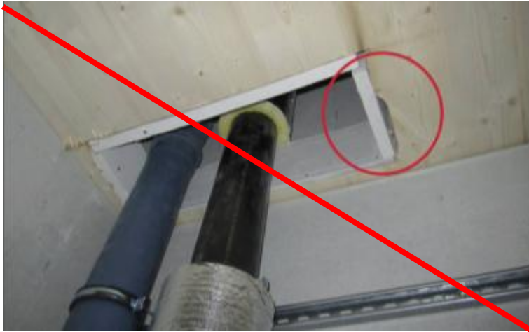
Figure 80: Installation of a reveal covering not over its entire surface
