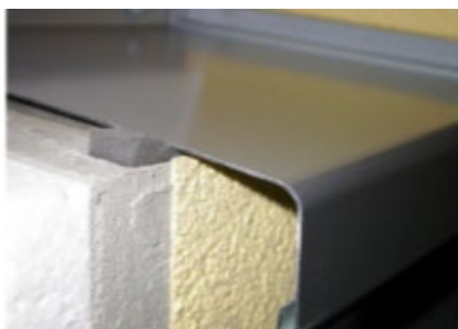
Figure 53: Horizontal joint under window sill towards facade surface with permeable sealing tape. Can also be executed in open form Source: [Österreichische Arbeitsgemeinschaft Fensterbank]
