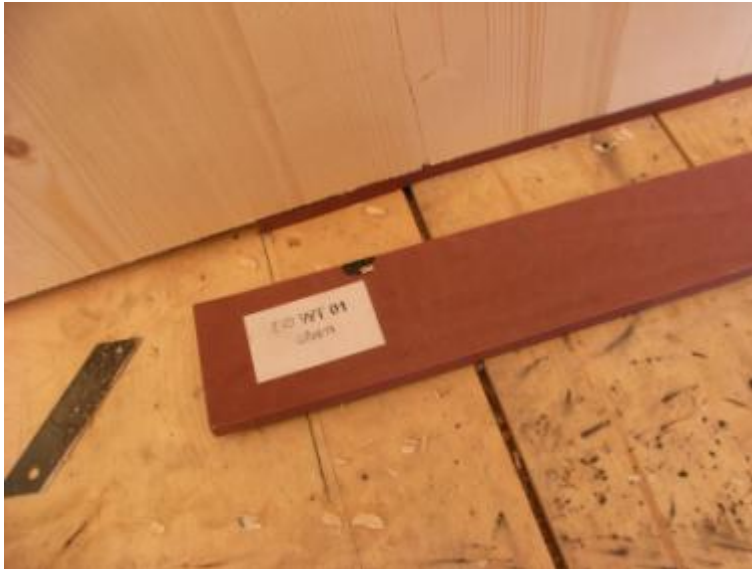
Figure 64: Sylomer supports in the padding support area for decoupling
