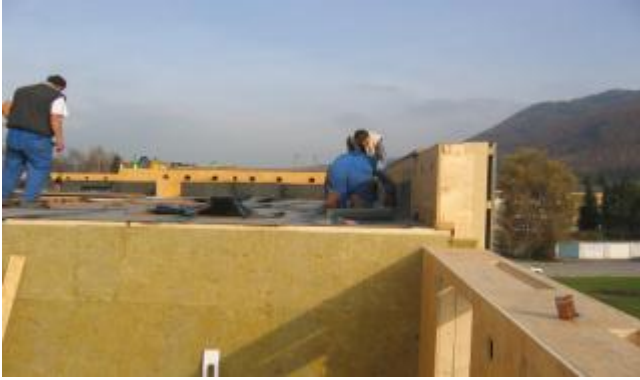
Figure 46: Vapor retarder (bituminous sealing) on a flat roof as a required weather protection
